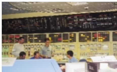
A section of the control room within the Gravelines nuclear power station operated by Electricite de France (Photo by Julie Morgan)
